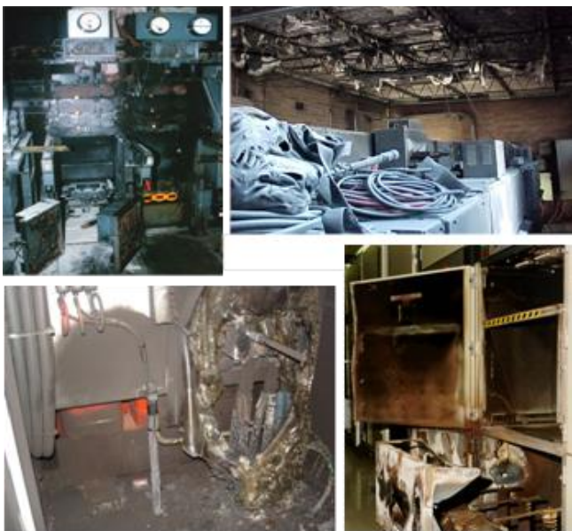
Fig5. Consequences of arcing faults
